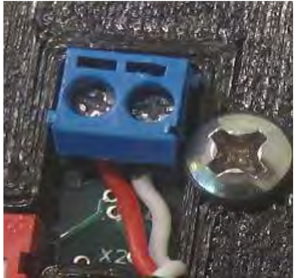
Valve Wiring -Red wire on Left
